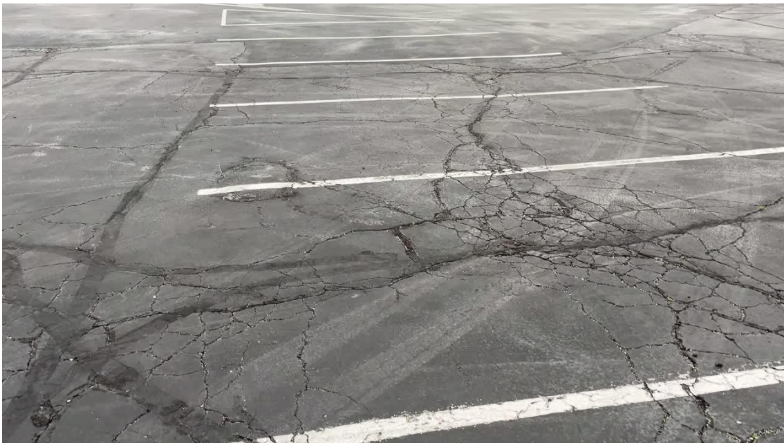
Interconnected cracking across a wider parking area, with both linear and fatigue-like distress visible.
