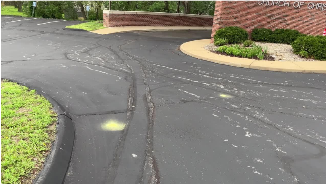
Long working cracks and prior repair lines near the building drive lane.
